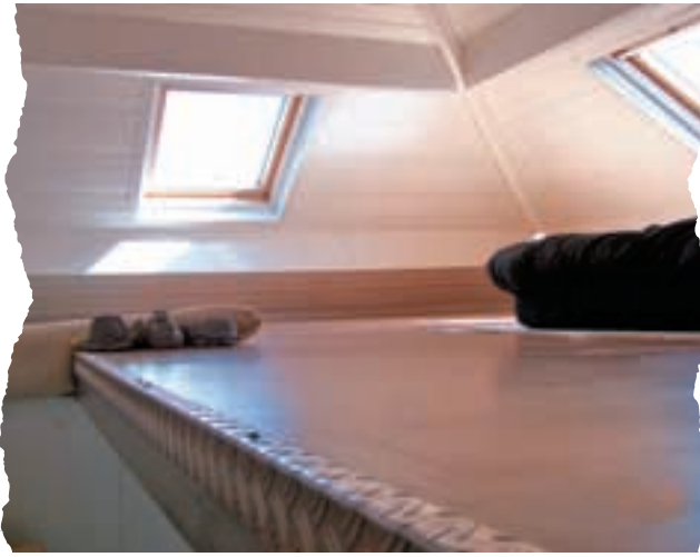
The ceiling in this loft conversion was about 3ft from the floor and the space had no safe stairs access.
